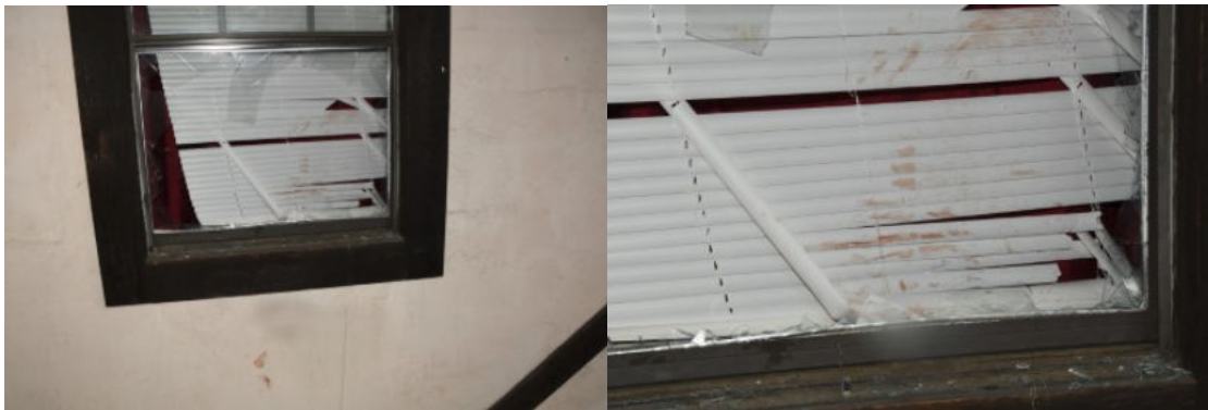
Broken window of Apartment A-8
