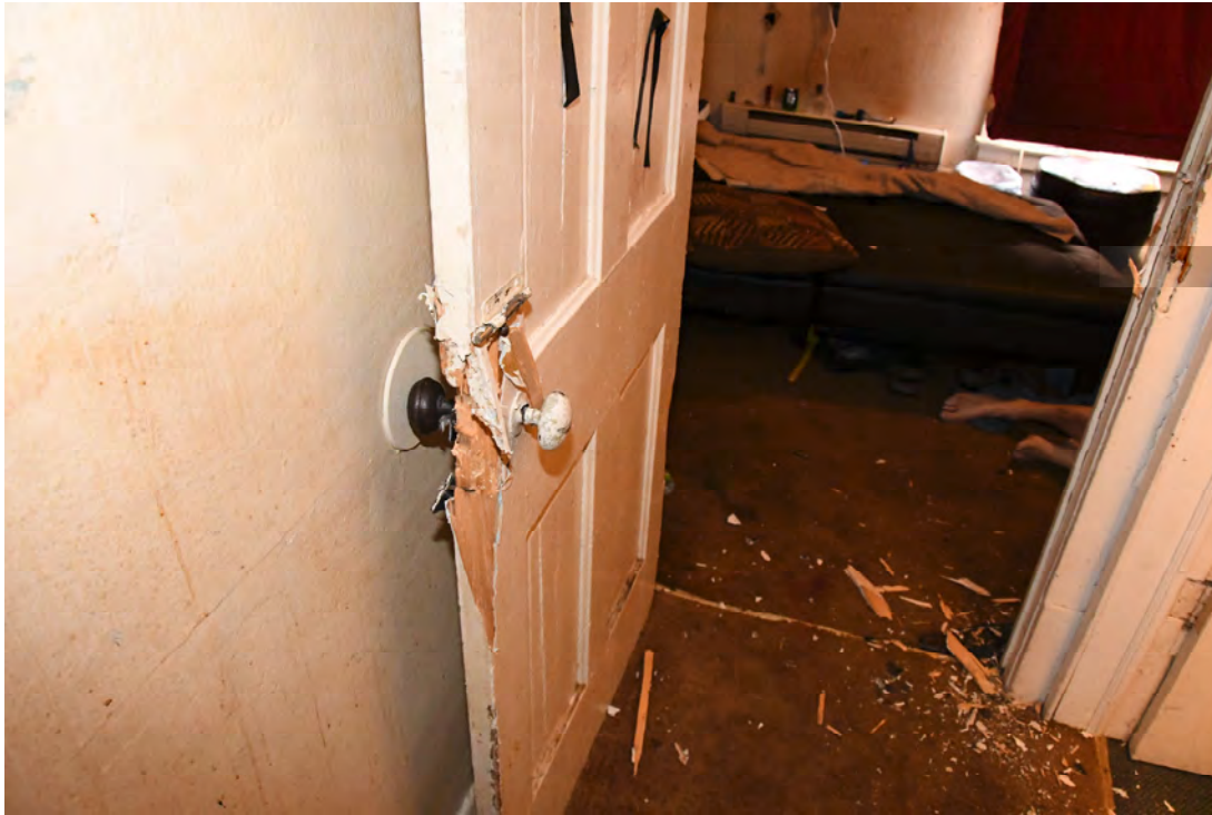
Damaged Bedroom Door
