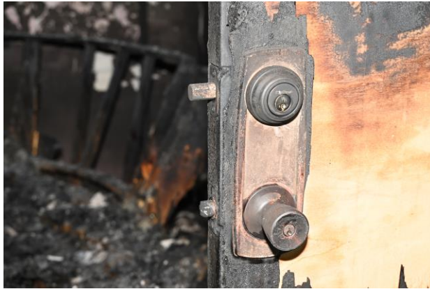
Image 2. Extended deadbolt on wooden door into main residence
