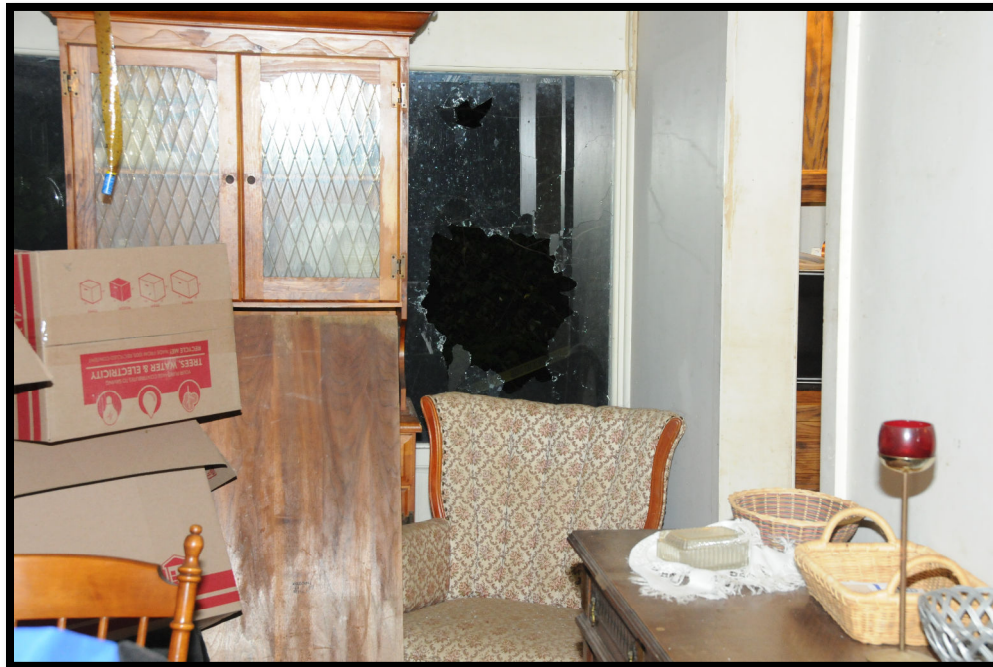
(Window shot out on west side of the house)
