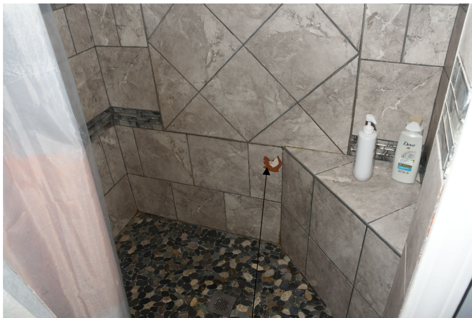
(damaged tile in master bath)
