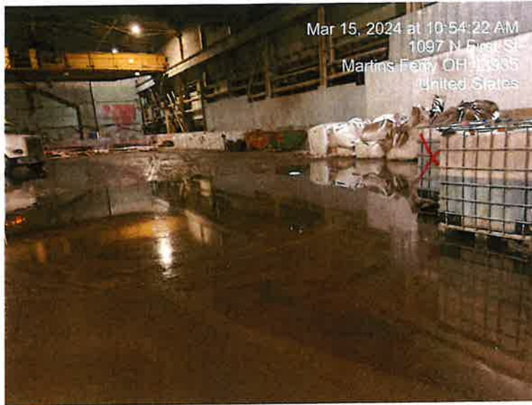
Liquid waste outside containment
