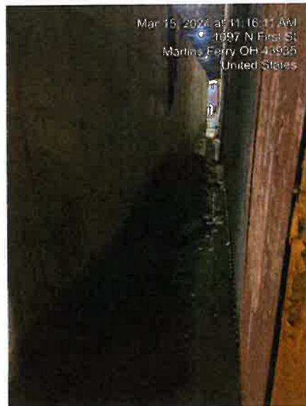
Waste behind bins
