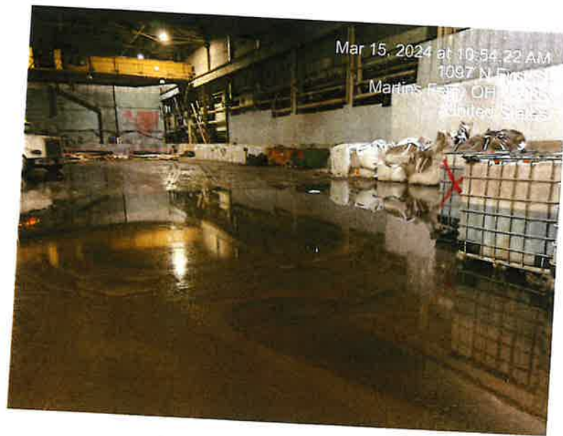
Liquid waste outside containment
