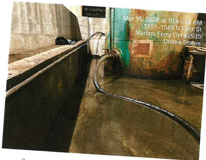
Secondary containment area for the south unloading area
